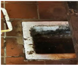
Photos: Clogged floor drains, April 16, 2024.
