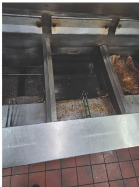
11/4/2025: Broken fryer- only the middle section works, and the oil is black, causing excessive smoke exposure, which is a health hazard.
