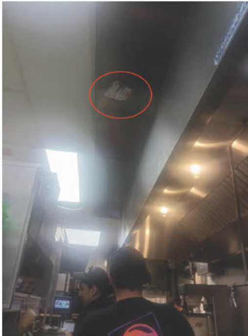
9/6/24: This photo shows the stickers that our coworkers placed on the ceiling to try to block the water leaking through the ceiling
